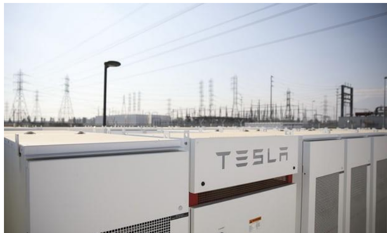
Fig. 14. Tesla’s Mira Loma substation in southern California
